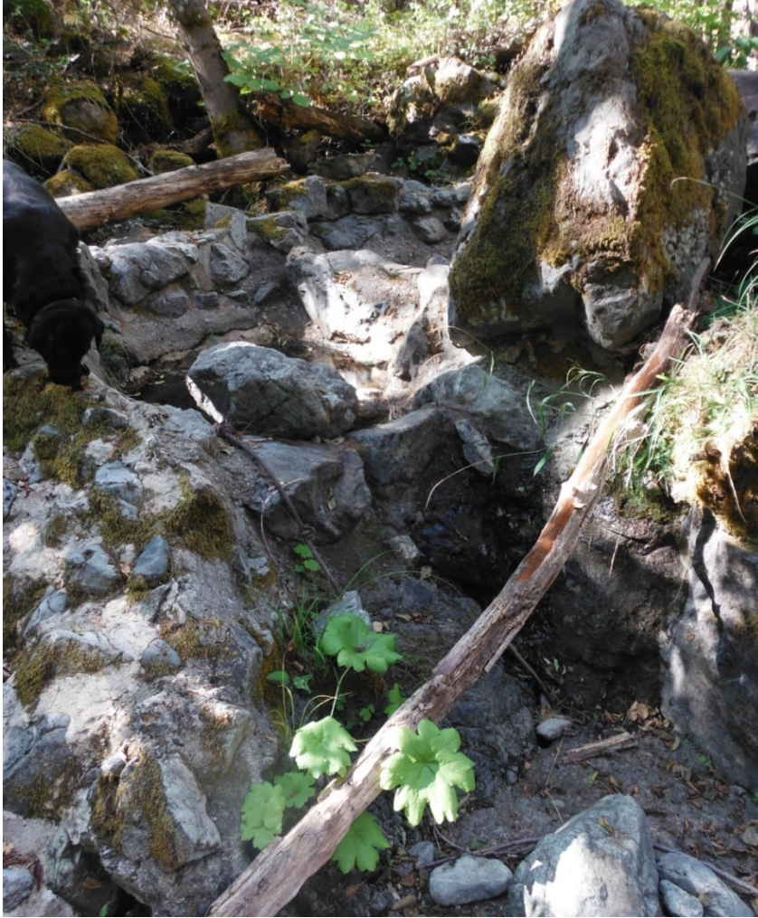
Figure 13. The Upper Tule Creek Diversion. Diversion structure and diversion pipe on the far right side of the photograph (a) and the fish passage structure (b).
