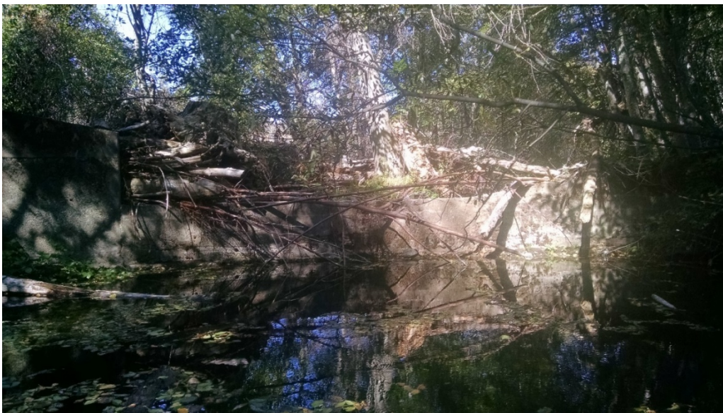
Figure 12. The lower diversion structure on Big Creek. on the primary channel looking downstream with the diversion gate and screen on the right (a) and on the secondary channel looking upstream (b).
