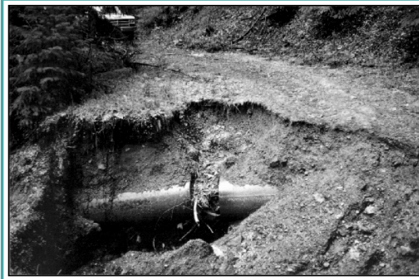
Problems identified on USFS road— Plugged culvert and blown crossing
